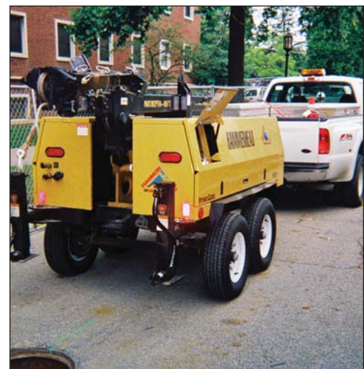
Top: Space was extremely limited. The pipe had to be held by crane on the jobsite. Bottom: The HydroGuide HG12 winch has a hydraulic deployable boom that only took 15 minutes to setup.
